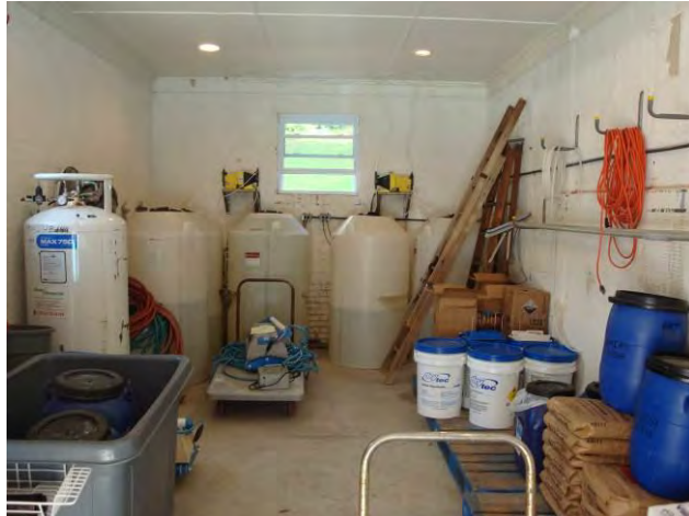
Image 82: Chemical Storage Room
