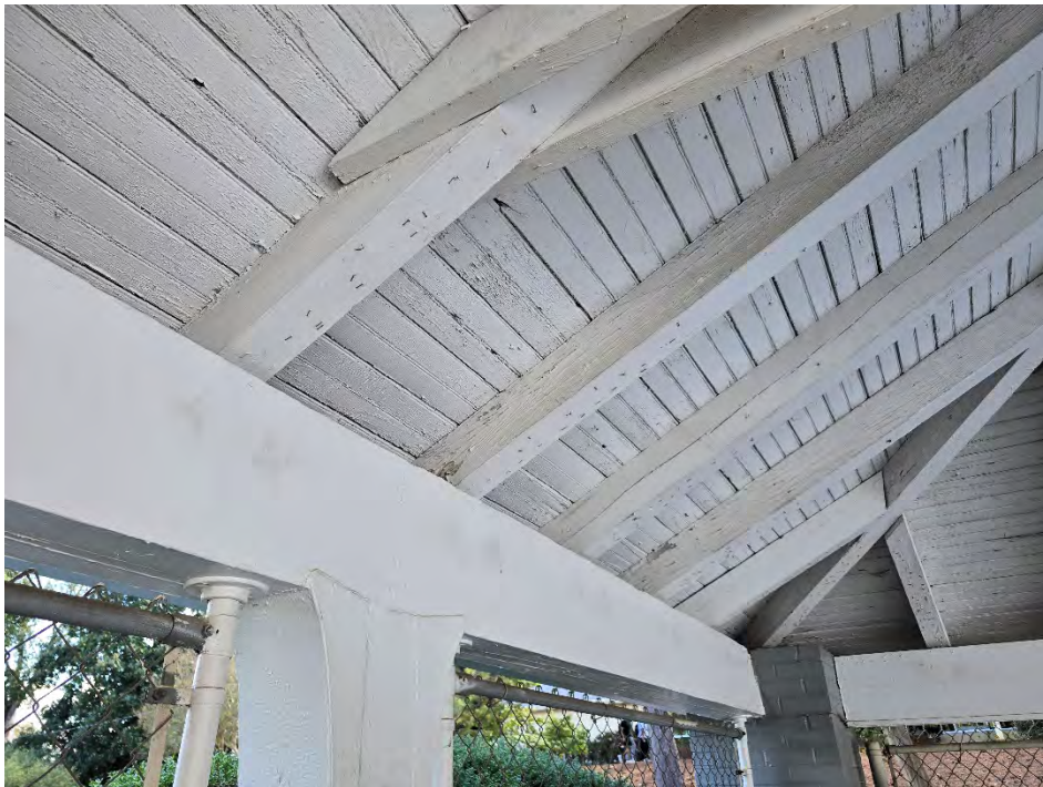
8. Exterior white damaged/peeling LBP on pavilion wood framing
