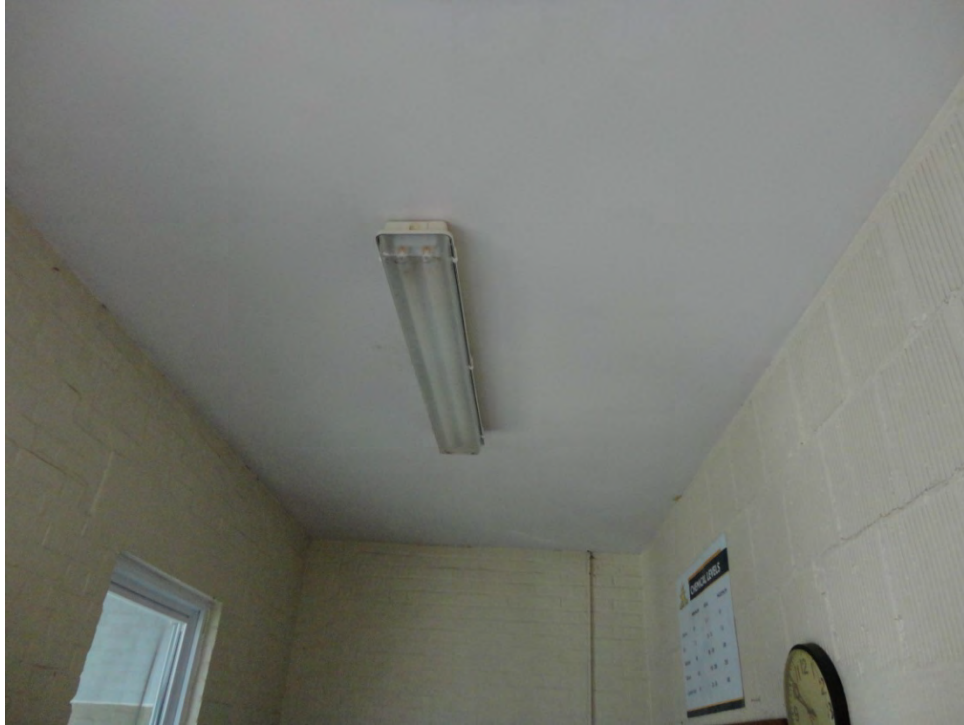
9. Typical mercury-containing fluorescent light bulbs in enclosed pool house structure.
