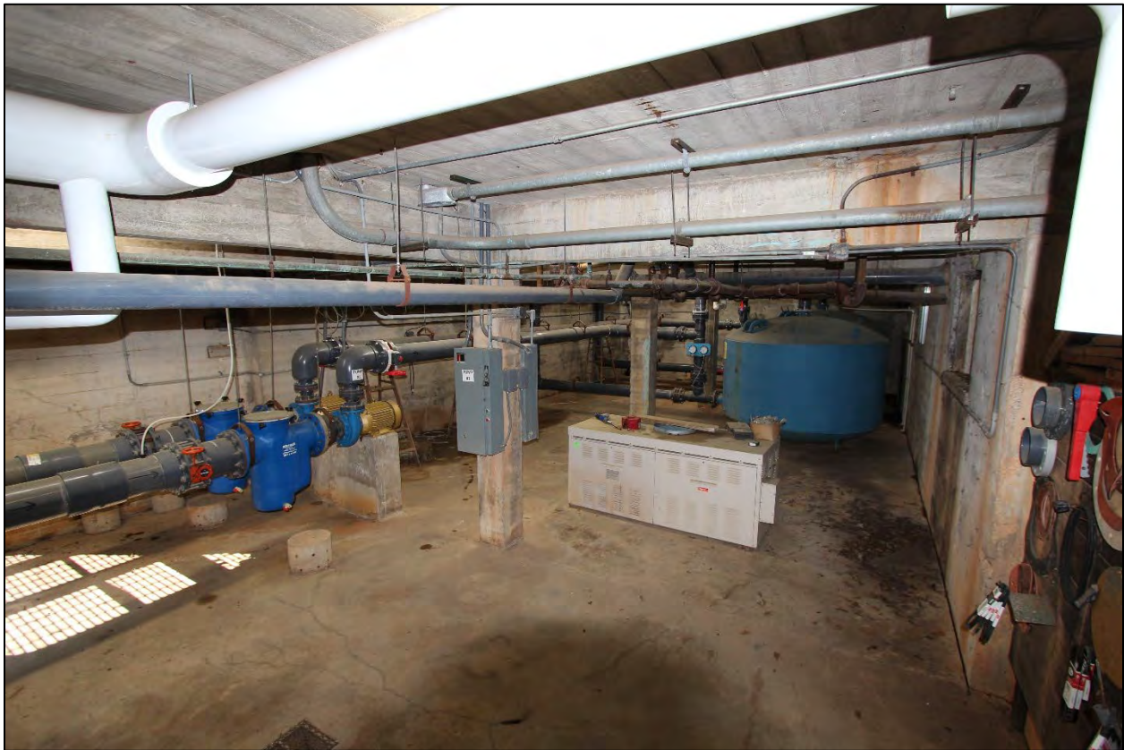
Figure 3.32 Pool House, basement, showing equipment, facing south.
