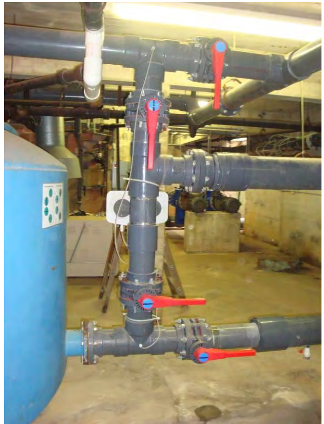
Image 72: Filter #1 Valve Manifold
