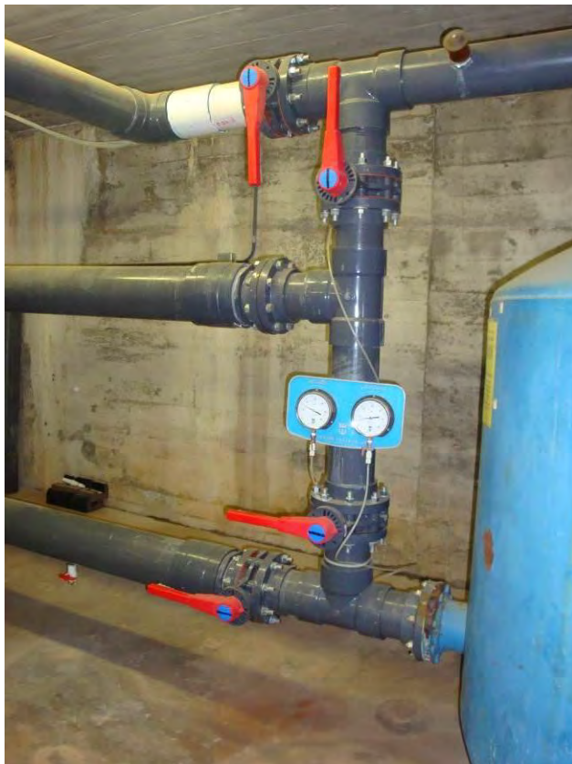
Image 71: Filter #2 Valve Manifold
