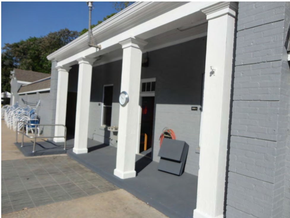
4. LBP in exterior white support columns in main structure.
