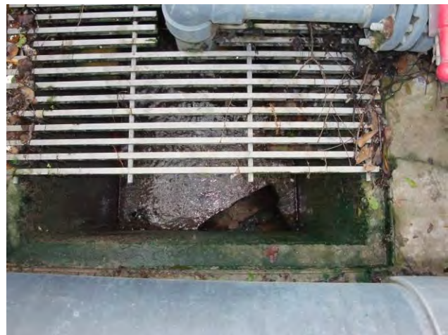
Image 38: Pool Drain Sump and Water From Under Pool
