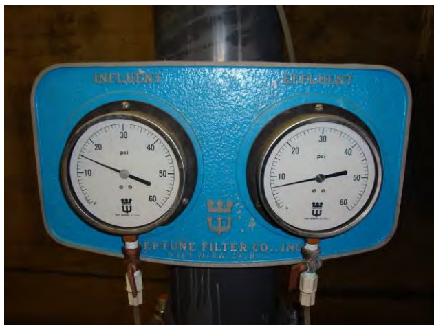
Image 59: Filter #2 Gauge Panel
