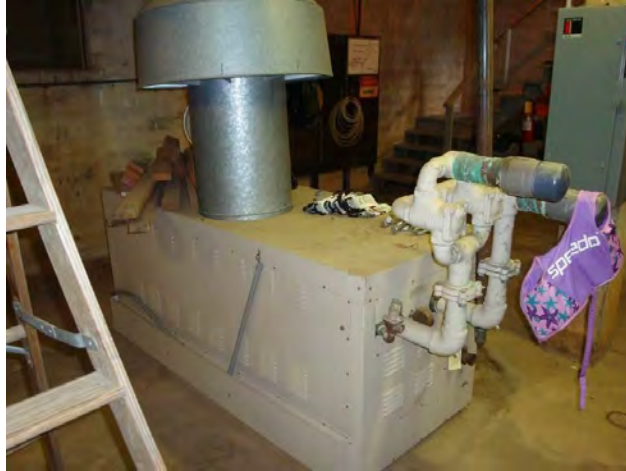
Image 89: Pool Heater and Piping
