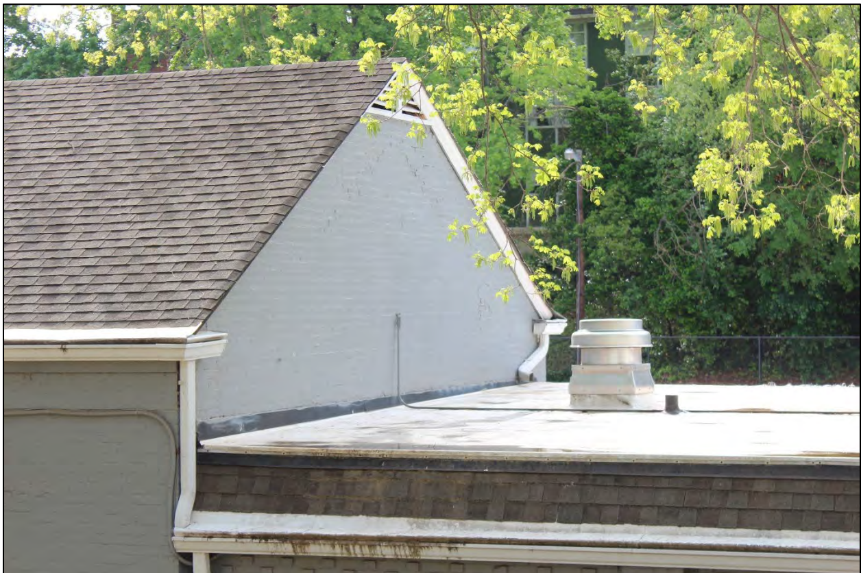
Figure 3.7 Pool House, ghost mark of old roofline, facing east.
