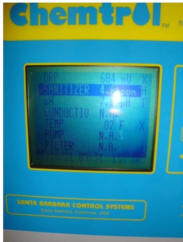
Image 85: Chemical Controller Display
