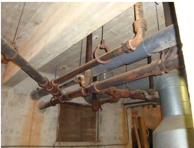
Image 62: Filter Backwash Piping
