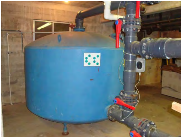
Image 55: Pool Filter Tank #1
