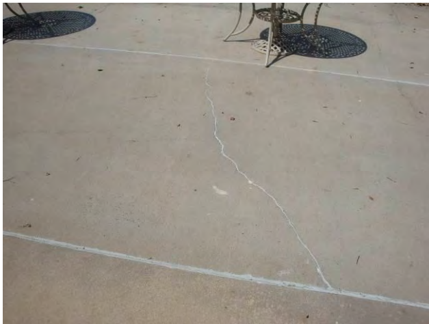
Image 28: Deck Cracks and Sealant
