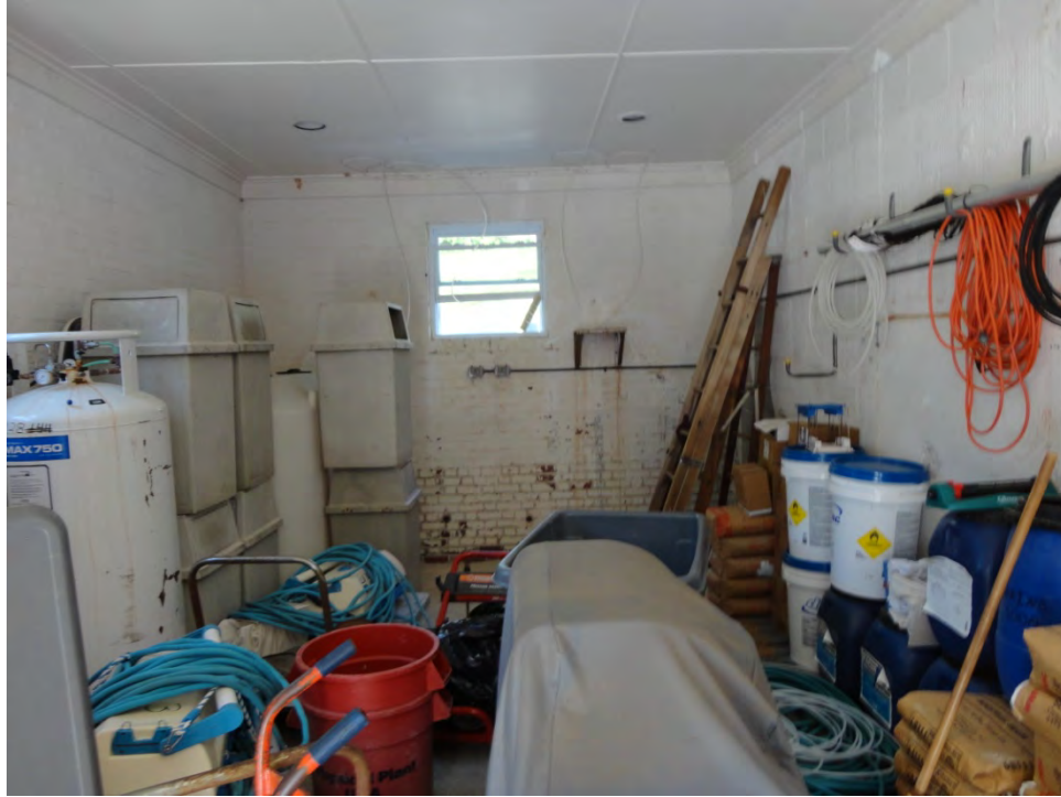
5. LBP in interior white brick walls in Storage Room 15.
