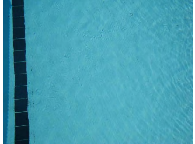
Image 4: Cracks in the Bottom of the Pool
