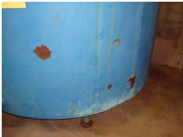
Image 57: Filter Tank Corrosion
