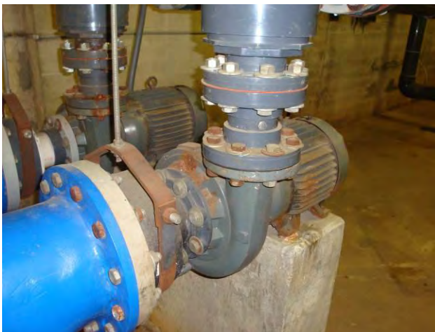
Image 52: Recirculation Pump with No Gauges
