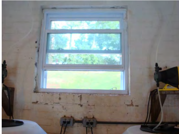
Image 78: Chemical Room Windows Open For Ventilation
