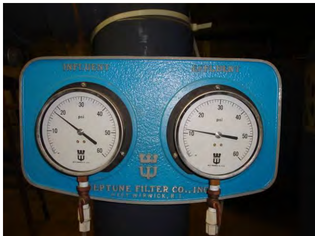
Image 61: Filter #1 Gauge Panel
