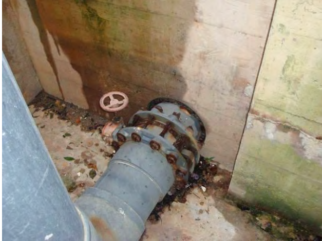
Image 69: Main Drain Valve
