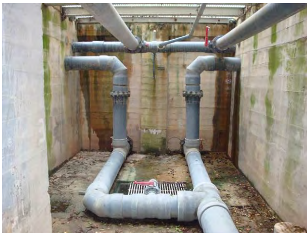
Image 37: Water Stains on the Walls
