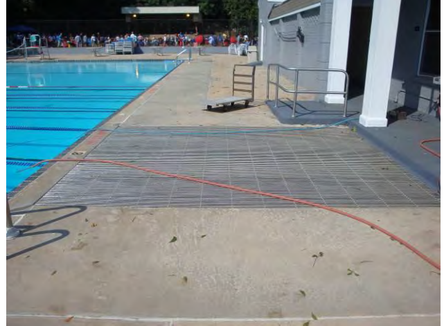
Image 27: Grating Over Below Grade Piping and Pool Mechanical Area
