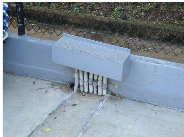
Image 17: Underwater Light Junction Box
