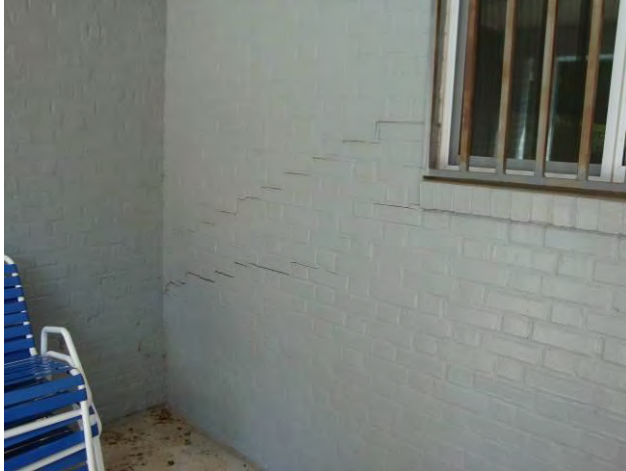
Image 94: Cracks and Settling in Concession Area
