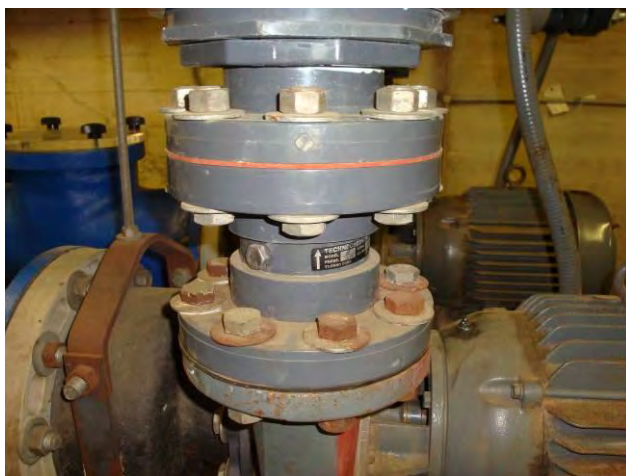
Image 73: Recirculation Pump Check Valve
