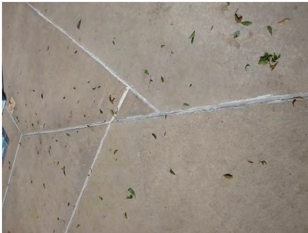
Image 24: Deck Cracks and Sealant
