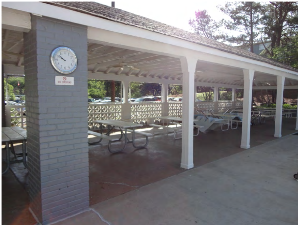
6. LBP in white support columns and ceiling in shade pavilion.
