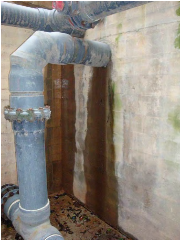
Image 39: Water Stains on the Walls
