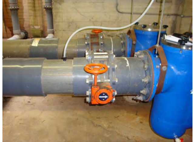
Image 70: Recirculation Pump Suction Isolation Valves
