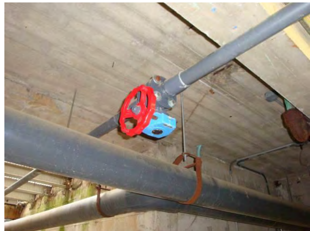
Image 91: Manual Fill Valve
