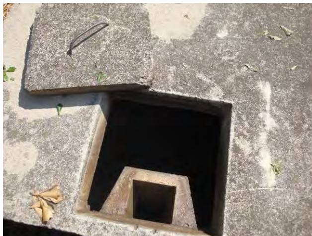
Image 65: Backwash Holding Tank Access Hatch
