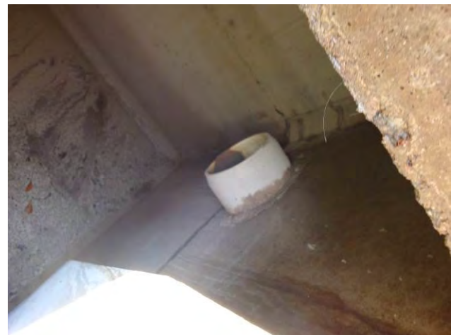
Image 66: Backwash Holding Tank Interior
