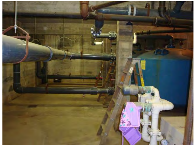
Image 42: Mechanical Room Piping & Hangers
