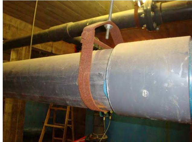
Image 44: Corroded Clevis Hanger
