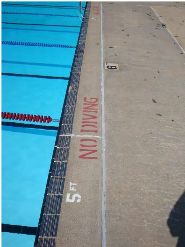
Image 9: Perimeter Overflow Gutter
