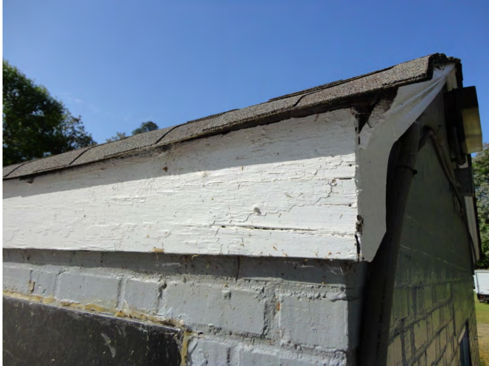
7. LBP in exterior white fascia board in main enclosed structure.
