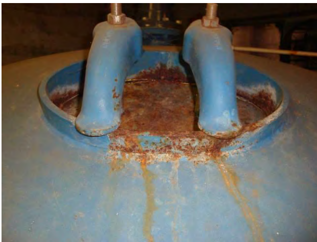
Image 58: Corrosion at Filter Manway
