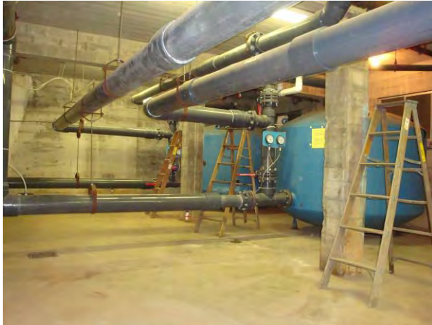
Image 43: Piping To/From Filters
