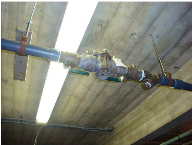
Image 90: Fill Line Backflow Preventer
