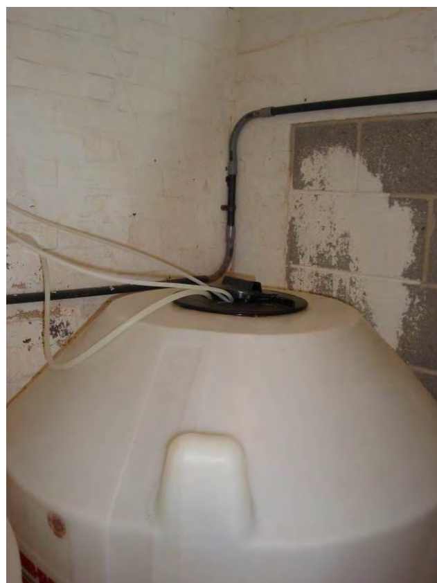
Image 76: Liquid Chlorine Storage Tank
