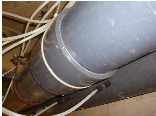
Image 46: Chemical Injection Points & Piping Leak
