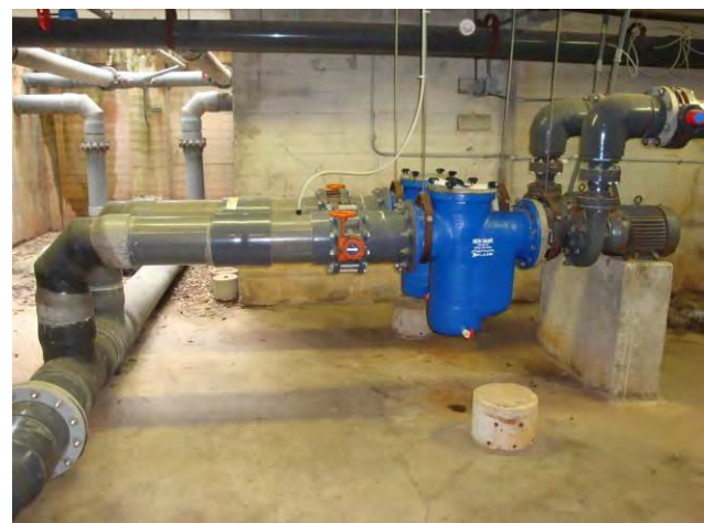
Image 50: Recirculation Pumps and Hair and Lint Strainers
