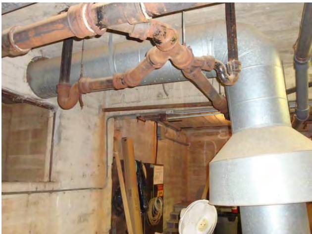
Image 88: Pool Heater Venting
