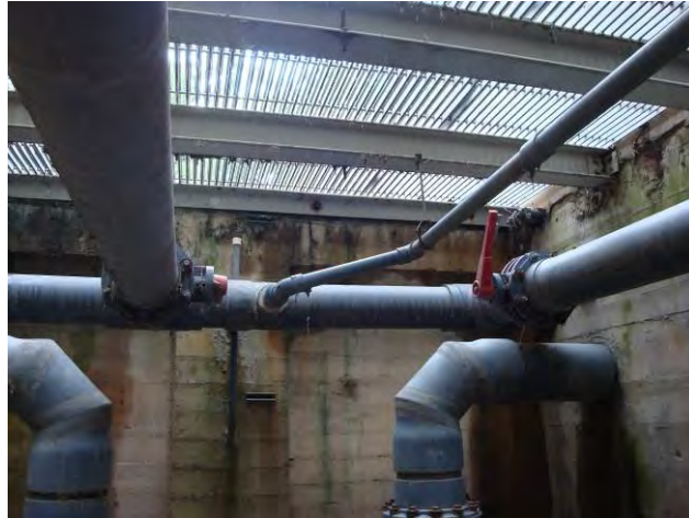
Image 92: Fresh Water Fill Connection to Pool Return Piping
