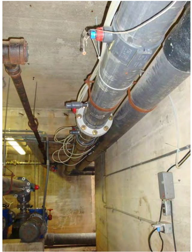
Image 40: Pool Return Pipe and Leak
