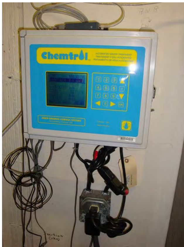
Image 84: Water Chemistry Controller
