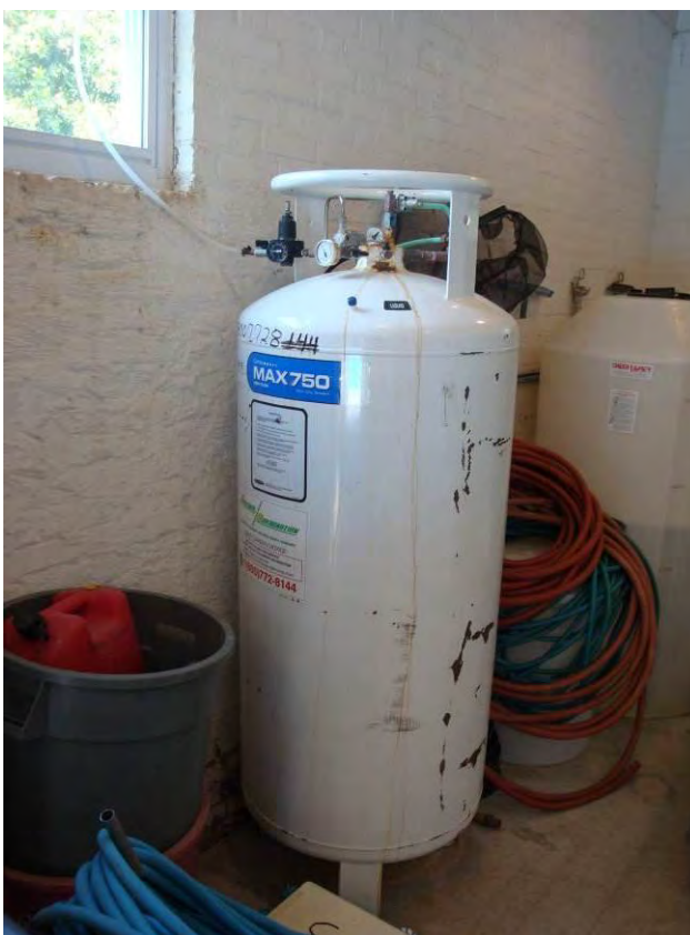
Image 77: 750 lb Carbon Dioxide Storage Tank
