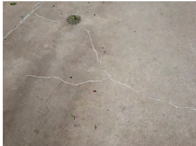
Image 25: Deck Cracks and Sealant
