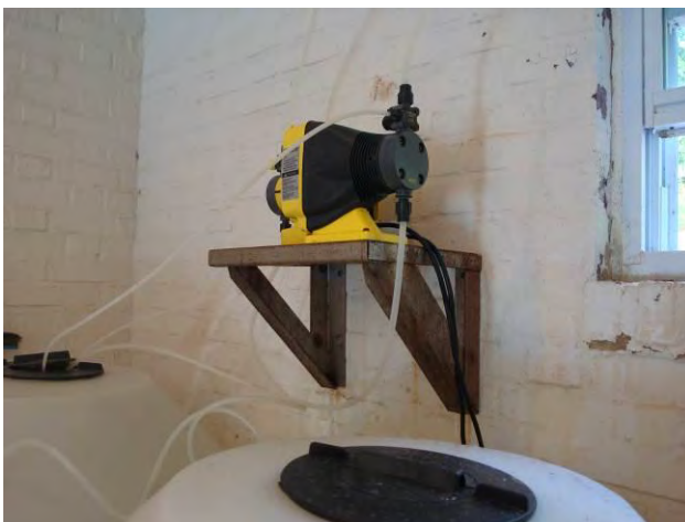
Image 75: Chlorine Pump and Shelf
