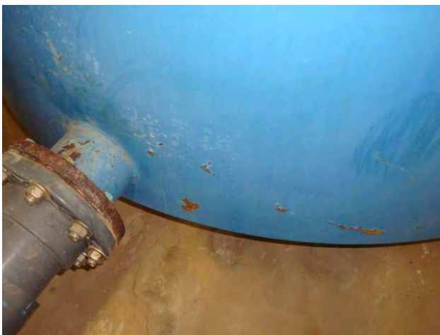
Image 60: Filter Tank Corrosion
