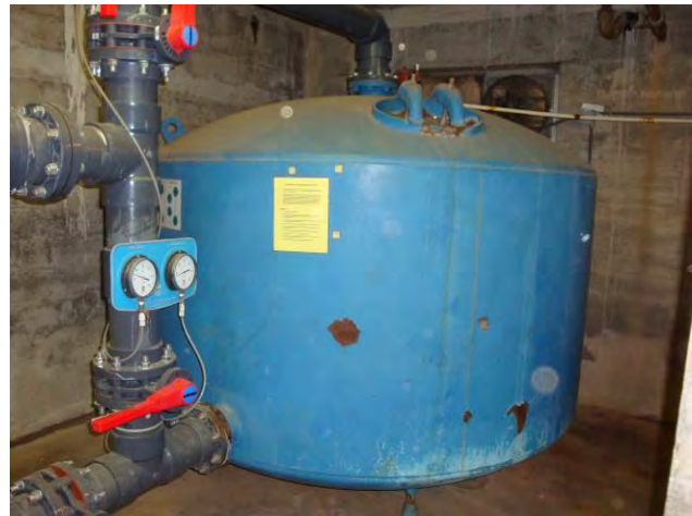
Image 56: Pool Filter Tank #2
