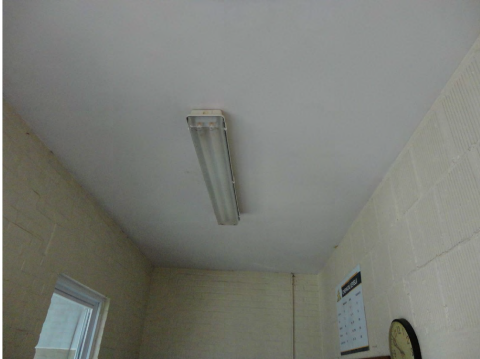
9. Typical mercury-containing fluorescent light bulbs in enclosed bathhouse structure.
