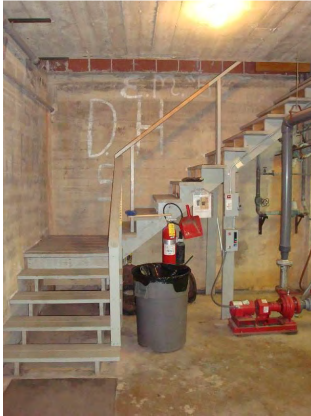
Image 93: Pool Mechanical Room Access
