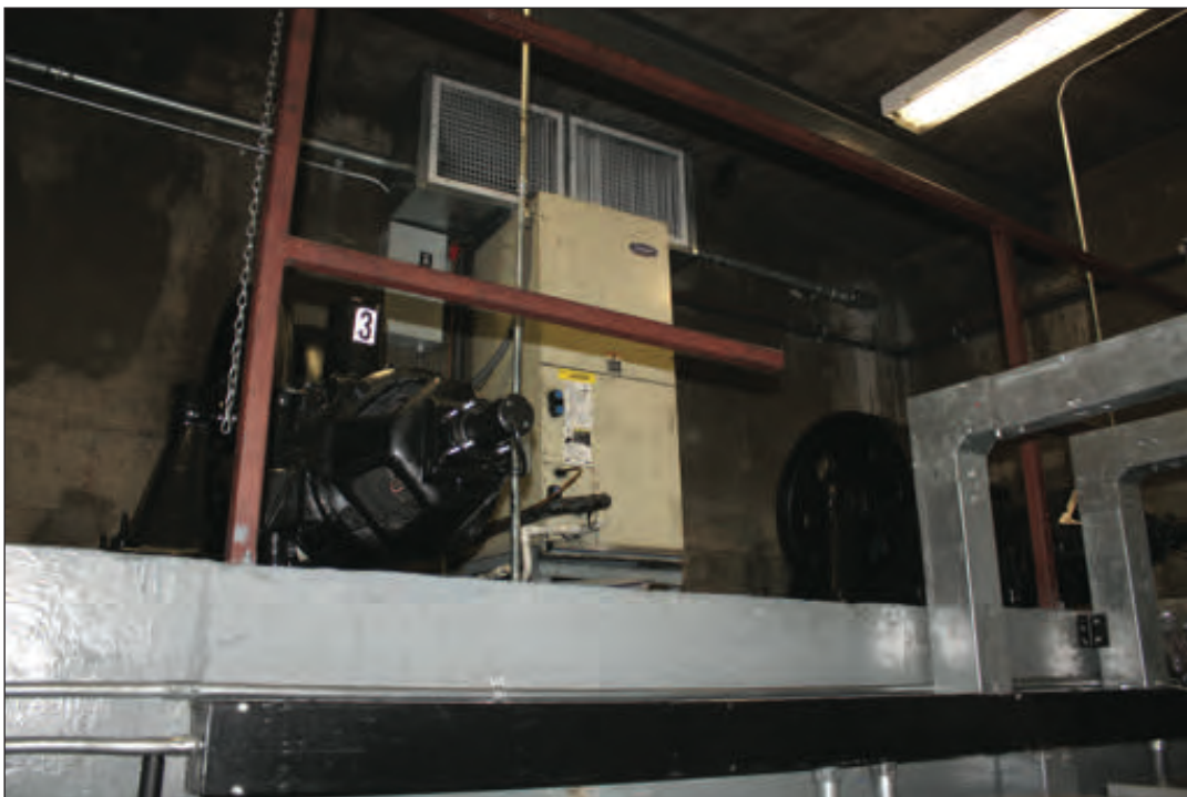
C. Sixth Floor Elevator Machine Room
