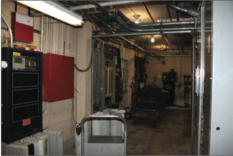
A. Equipment Room, View 1
