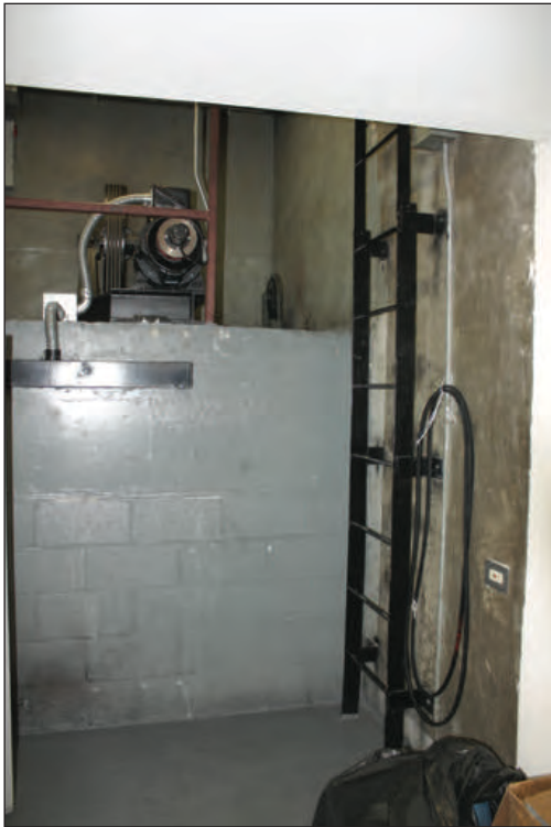
A. Rooftop Elevator Machine Room Interior
