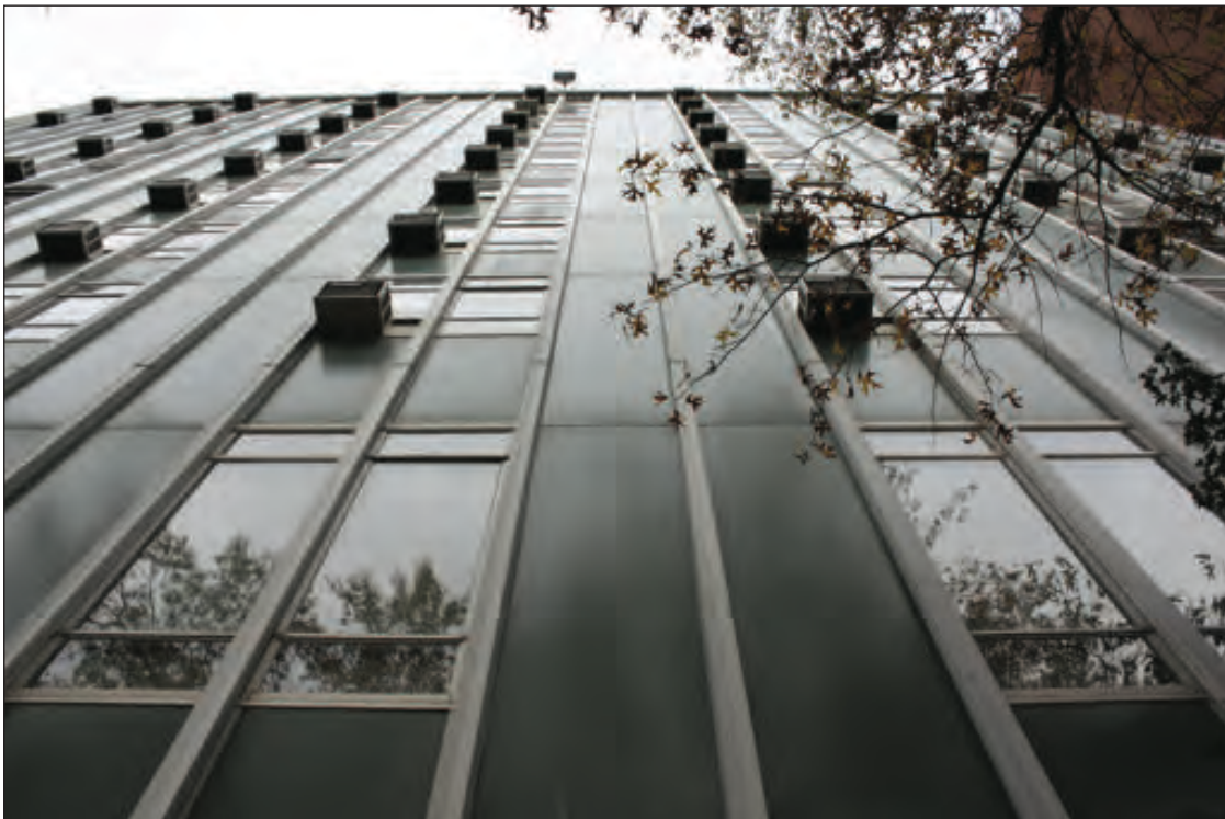
B. Enamel Panels on South Tower
